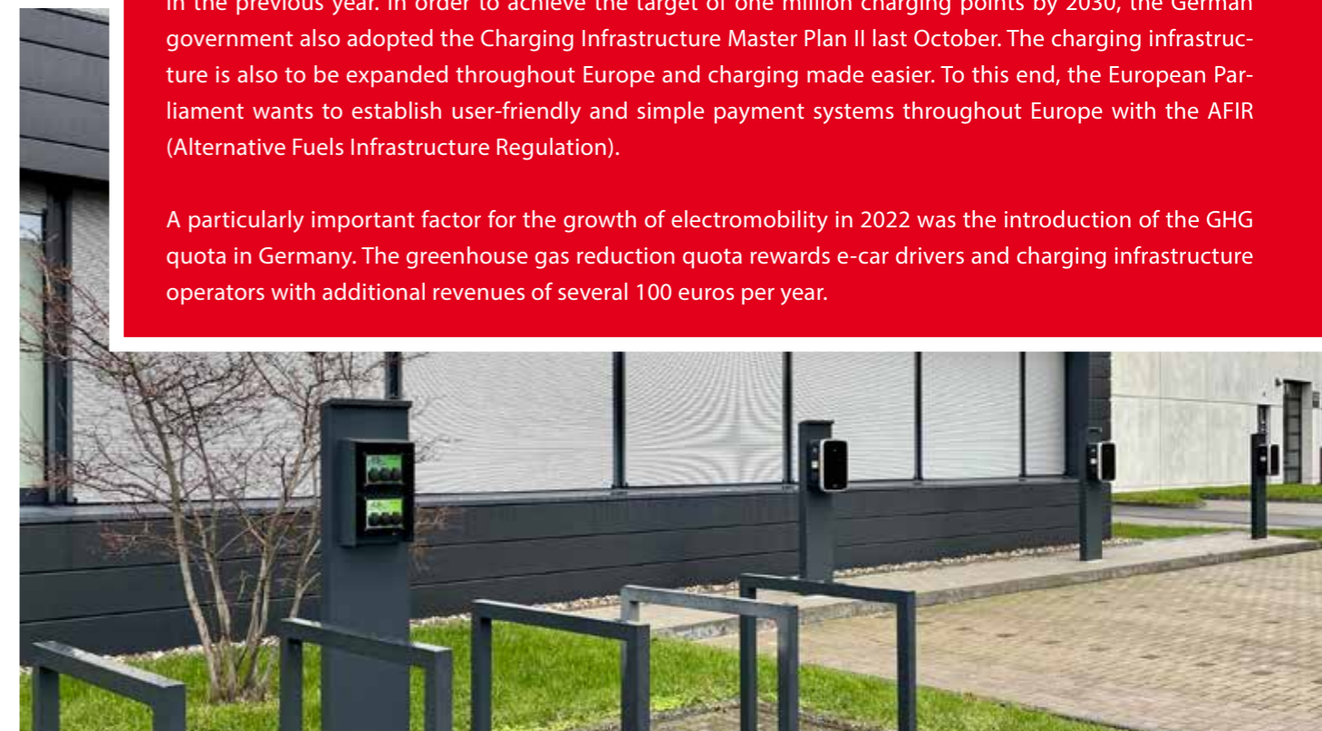
Charging stations for electric mobility. EK focuses on sustainable solutions in its offering.
